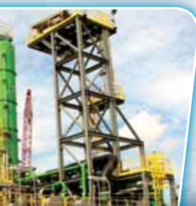
FPSO Esprito Santo (Sea Water Treatment Module)
