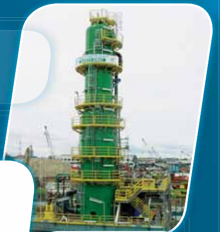
FPSO Marlim Sul (Injection Module Treatment)
