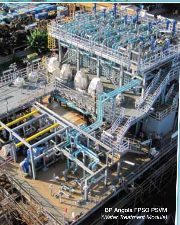
FPSO Cascade/Chinook Fields (Power Generation Module)
