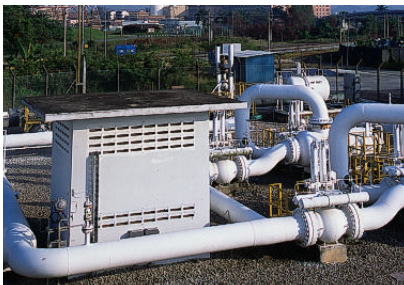
PGB's meter station for Connaught bridge Power Plant in Kapar, Klang. Stesen memeter PGB bagi Loji Janakuasa Connaught Bridge di Kapar, Klang.
