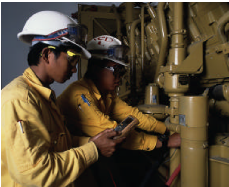
Electrical technicians, Abdul Halim bin Abdullah and Mohammad Hidher bin Othman checking battery voltage at a generator set at GPP4.
