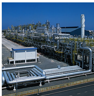
A bird's eyeview of the Cogen Unit which houses all six Gas Turbines and Heat Recovery Steam Generators (HRSG) of CUF Kertih.
