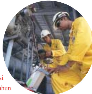
Top/Atas : Online control valve calibration at Compressor House Kawalan 'online' kaliber injap di Rumah Pemampat
