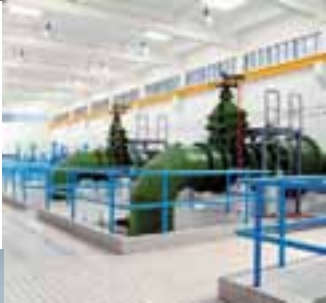
Treated Water Pumps
