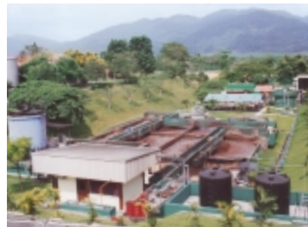
Waste Water Treatment Plant in Chembong / Loji Pemulihan Air Sisa di Chembong
