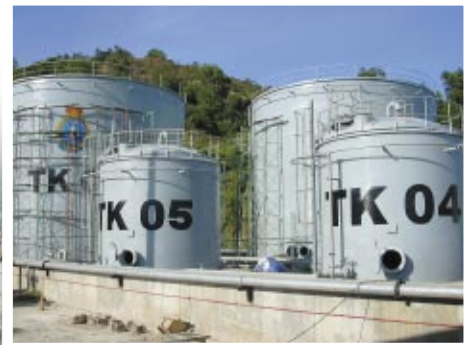
Diesel and Jet Fuel Tank farm for Sepangar Naval Base by Muhibbah Petrochemical Engineering Sdn Bhd
