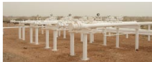
Oil gathering manifolds for Field Surface Facilities Project, Sudan by Muhibbah Petrochemical Engineering Sdn Bhd
