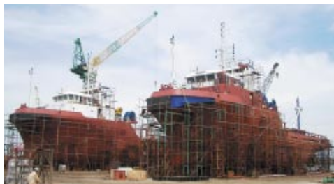
Fabrication on Work of Offshore Supply Vessel By Muhibbah Marine Engineering for Oil & Gas Industry
