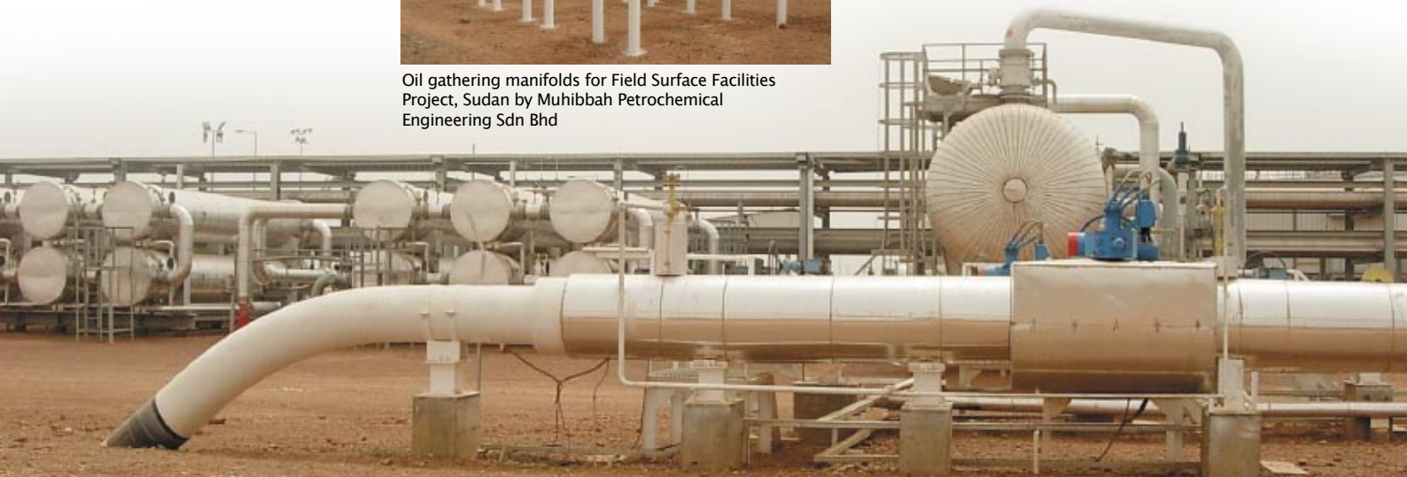
Oil receiving facilities for Difra project in Sudan completed by Muhibbah Petrochemical Engineering Sdn Bhd
