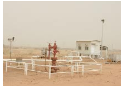
Typical substation and piping for oil well, completed by Muhibbah Petrochemical Engineering Sdn Bhd
