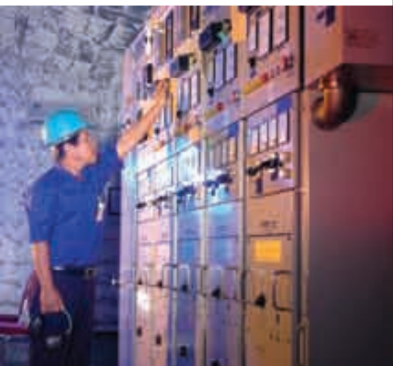
Monitoring powerhouse operations at PT Koba Tin, Indonesia.
