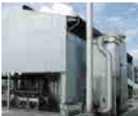
Gas cleaning plant.
