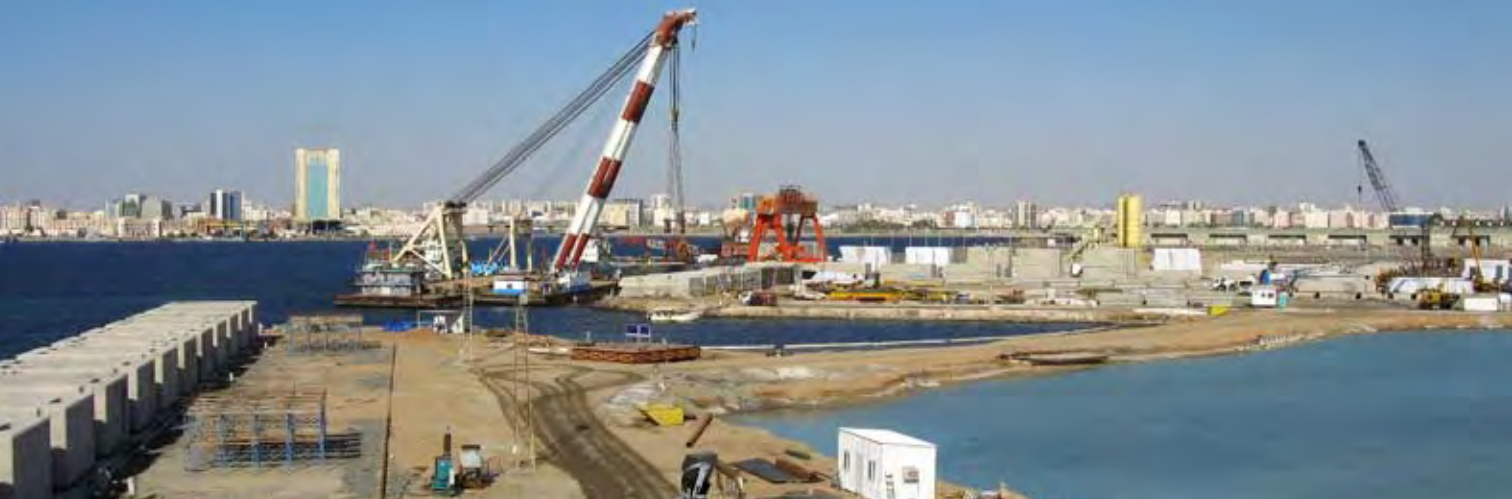
Construction of the new Red Sea Gateway Terminal at Jeddah Port, Saudi Arabia
