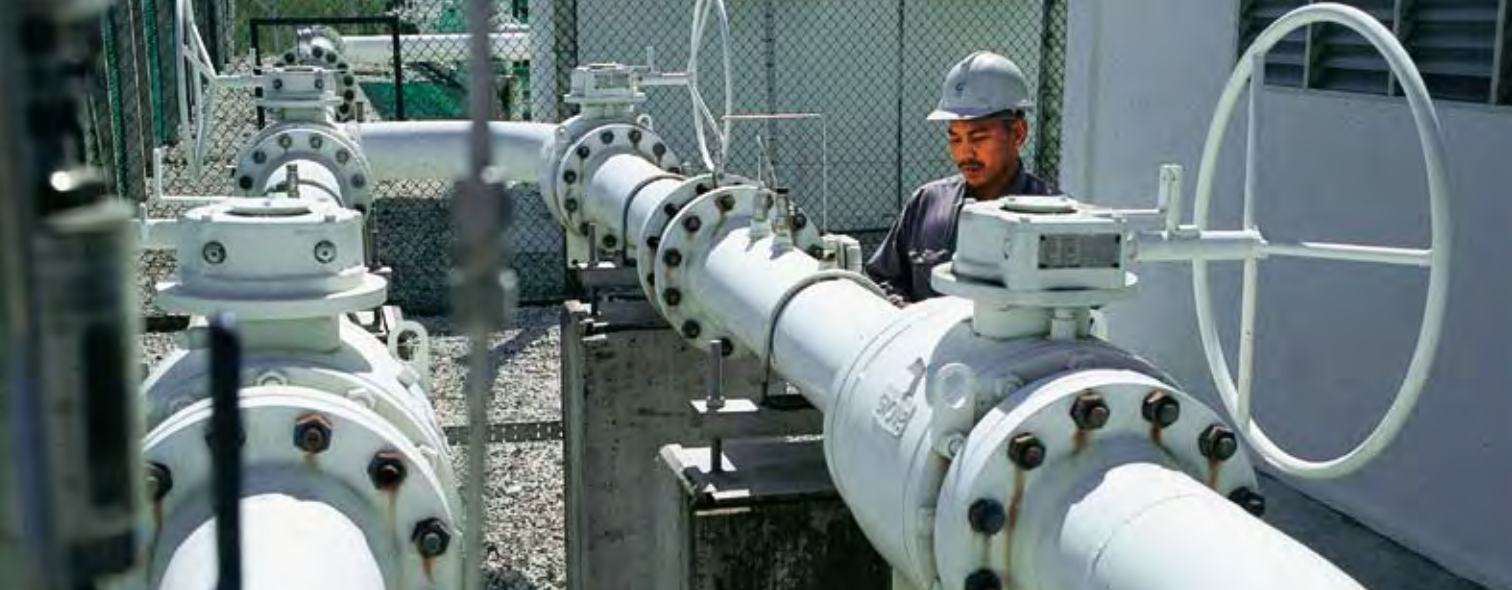
Gas Malaysia's odoriser station
