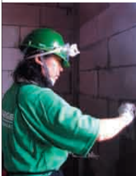
A volunteer from Lafarge Malayan Cement helping to rebuild homes for the devastated victims. The culture of caring for the communities provides sustainability to Lafarge's continuous growth.
