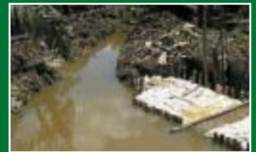
Fresh water from hills diverted for flushing of acidic water and irrigation to peat soils in Kebun Nilo
