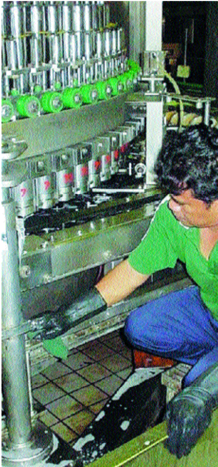
Thorough and regular checks on the canning line ensure optimum operational efficiency
