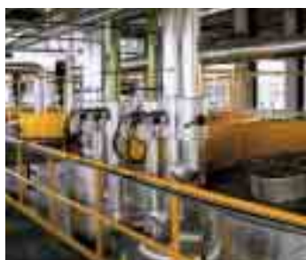
New plant in operation at Jomalina.
