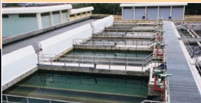
Bukit Badong Water Treatment Plant Phase 1 & 2 have a capacity of 800 mld. Loji rawatan air Bukit Badong Fasa 1 & 2 berkapasiti sebanyak 800 mld.
