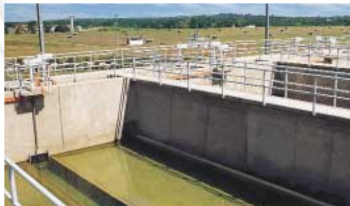
Filtration Tanks. Tangki penurasan.
