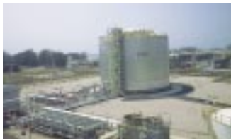
• Propylene tank & ancillary facilities.
