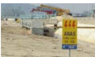
• Completed cabling work with cables signboard and cable bridge at the background.
