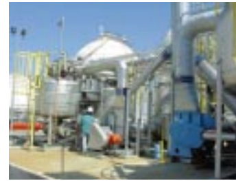
• State-of-art vapour emission control system.
