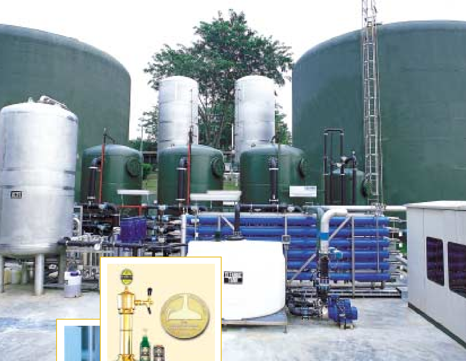
The newly installed water treatment plant.
