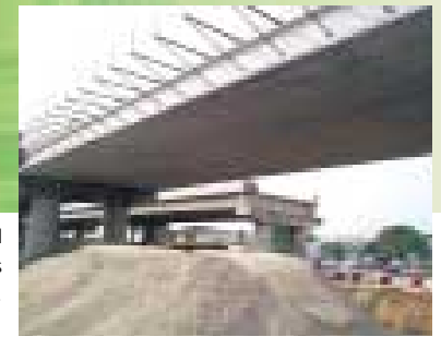
Excavation works for the 2nd phase of the PJS 8 underpass at Bandar Sunway.
